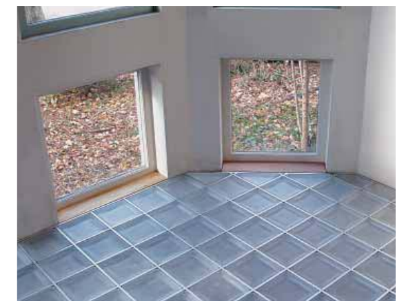
Pavers can be cut to turn non-square corners, as in this custom-designed floor.
